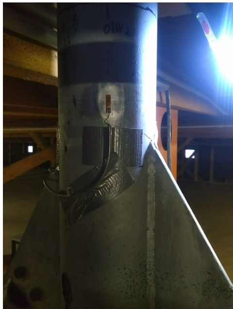
Figure 4.34 Tower-base bending loading measurement using strain gauge sensors.
